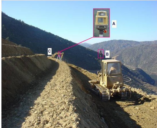
Figure 1 Construction of narrow terraces, using a laser system (Adapted from Guimaraens and Magalhães, 2006)
